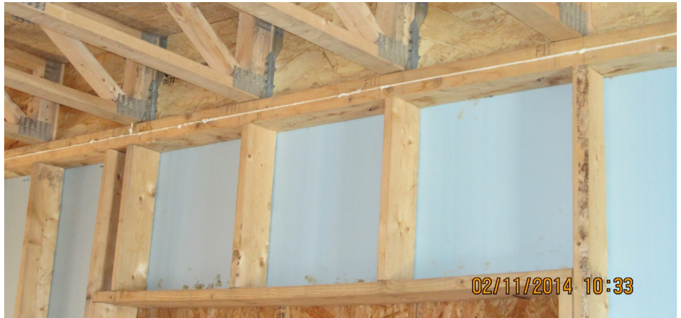
Figure 17. Double Rim Beam A rim beam configuration replaces window headers, leaving more room for insulation. Note joist hangers above opening and caulk to seal between plates.
