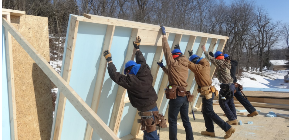
Figure 13. EP&B Wall Field-Framing. Note Top Plate End Gap to Tie into the Neighboring Panel.
