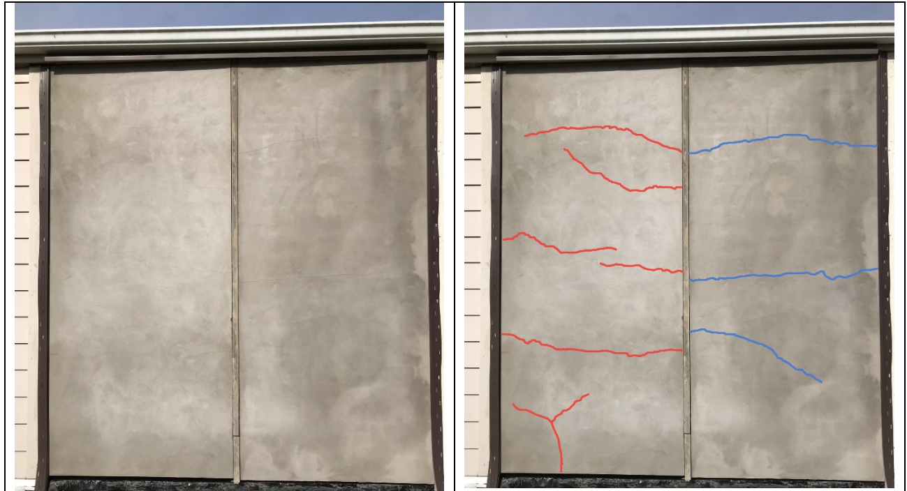
Figure 28. Cracking Observed in Outdoor Specimens
