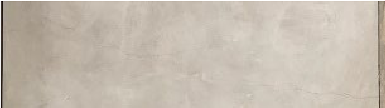
Above: 4-in. on center staples penetrating stud framing, lower set of cracks
