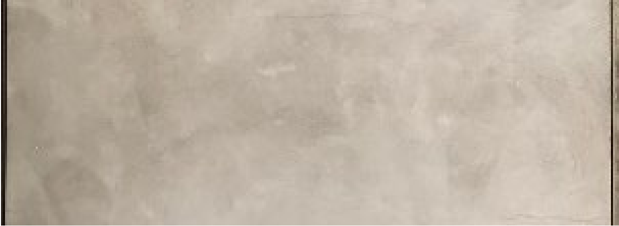
Above: 4-in. on center staples penetrating stud framing, upper set of cracks
