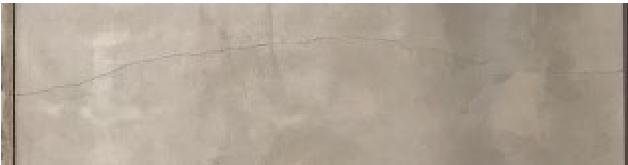
Above: 6x6 grid pattern with no stud penetration, upper set of cracks
