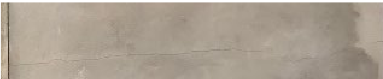
Above: 6x6 grid pattern with no stud penetration, lower set of cracks
