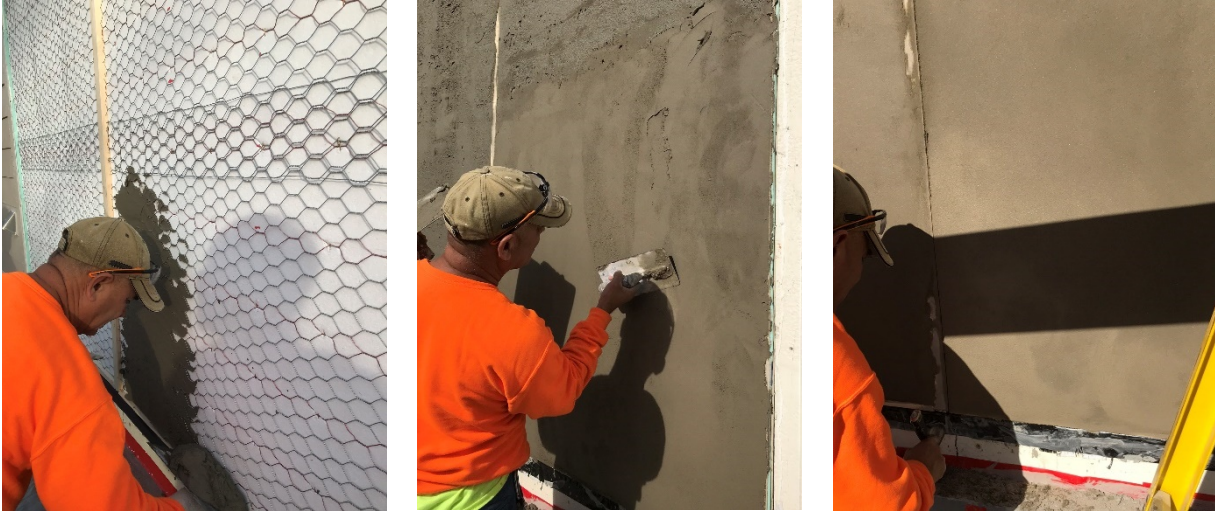
Figure 25. L to R: Initial Stucco Application, Surface Finishing, Scoring at Edges to Prevent Adhesion
