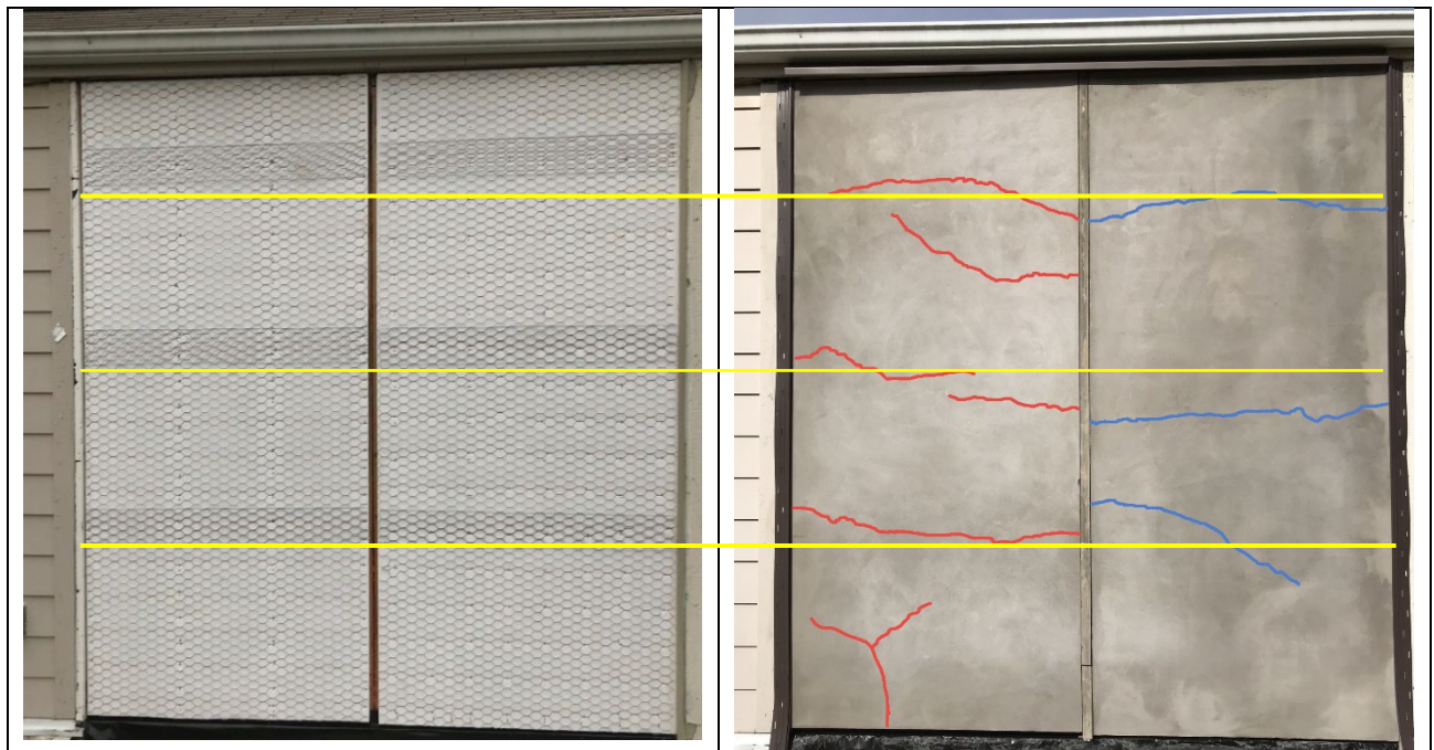
Figure 29. Outdoor Specimen Cracking with Reference to Lath Installation
