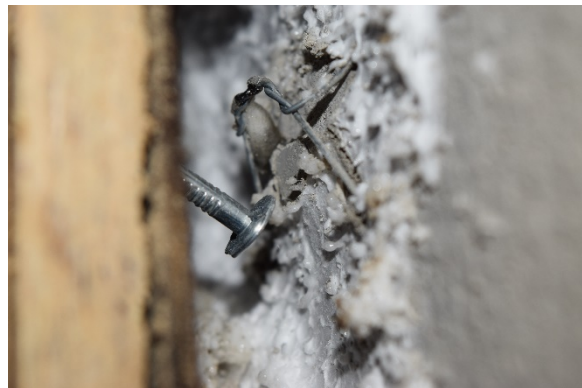
B. Failure Mode was a Combination of Nail Bending and Lath Wire Deformation
