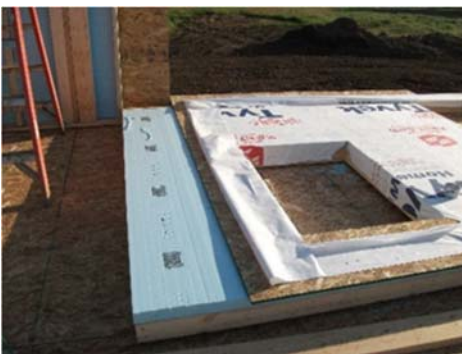
Two adjacent sections of wall must be planned to stagger the vertical joints of the rigid foam and OSB.
