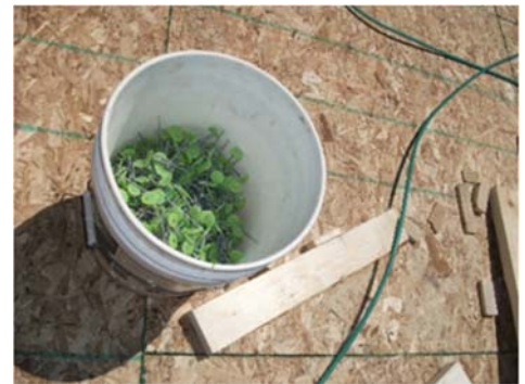
Cap nails can keep the rigid foam in place until the OSB is fastened over the top.
