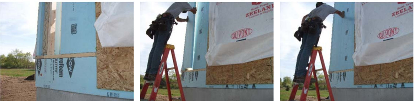
Fill in the EP&B components at the outside corners of the short wall and provide a continuous rigid foam layer.
