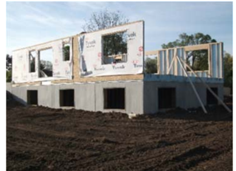
When adjacent wall panels are in place, fill in the EP&B layers as necessary: rigid foam, then OSB, then WRB.
