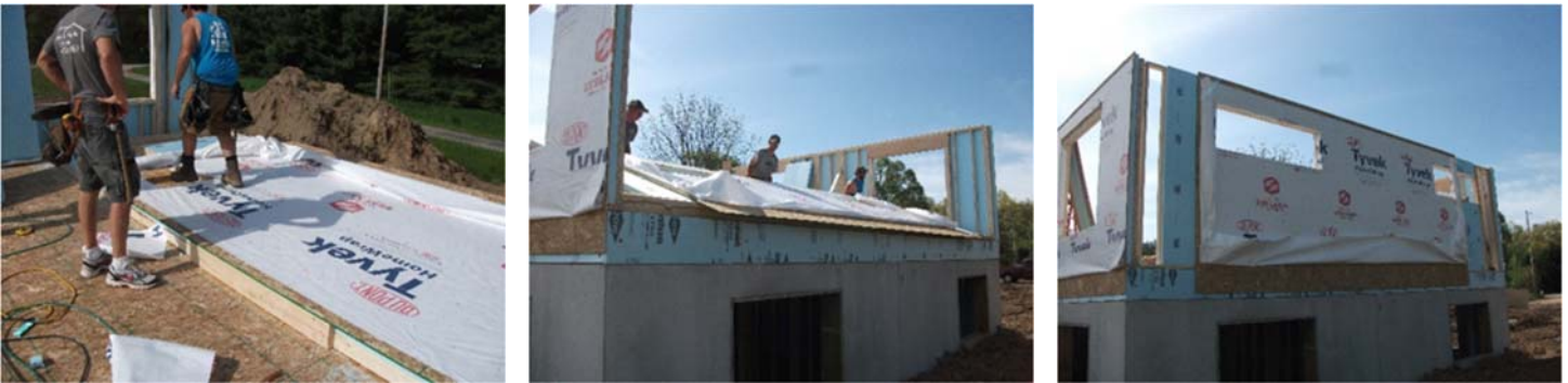
Raise the short wall and tie-in to the long walls on each side, with rigid foam and OSB gaps to allow maneuverability and connection, to be filled later from the exterior side of the wall.
