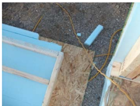
The gap provides a slot for the other wall's foam layer. Air-seal connection with caulk.
