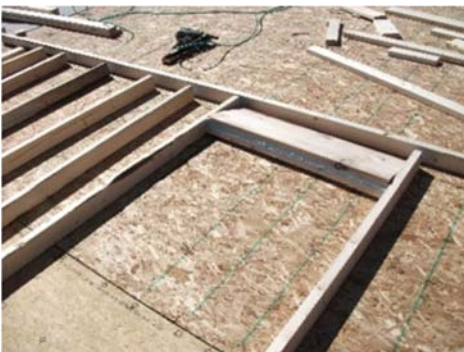
Position studs and headers according to layout markings on plates. Remember that all plates will be one dimension wider than studs, unlike what is shown here.
