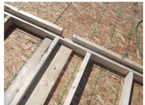
Leave gap in top plate for tying-in interior partition walls. Remember that all plates will be one dimension wider than studs, unlike what is shown here.
