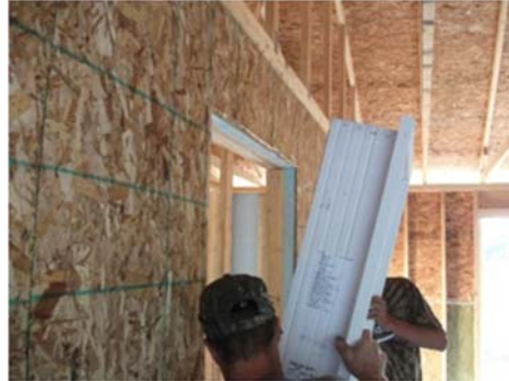
Tipping the door into place. Note that between the house and garage, the OSB was detailed as the air control layer.
