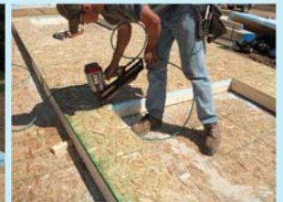
Nail OSB at top and bottom plates and use circular saw to cut OSB at opening.
