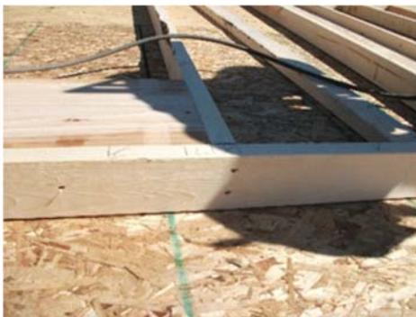
End-nail headers and studs. Remember that all plates will be one dimension wider than studs, unlike what is shown here.
