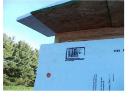
Ensure air-seal at sole plate. Here, the OSB will lap the rim for improved seal.
