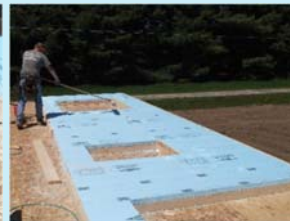
Sweep away debris and lay in OSB, careful to stagger joints vs foam.
