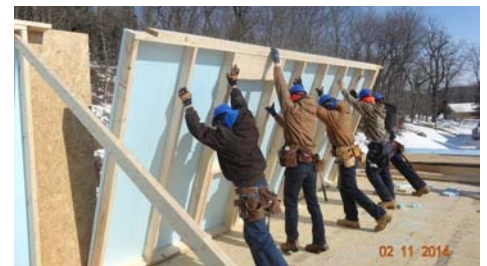
EP&B Wall Panel Erection —Note top plate end gap and sheathing overlap to tie into the neighboring panel.
