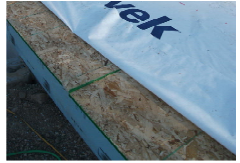
Staple WRB into place. Fold back and tack long edges that need to wrap down or around when the wall is later tipped up.
