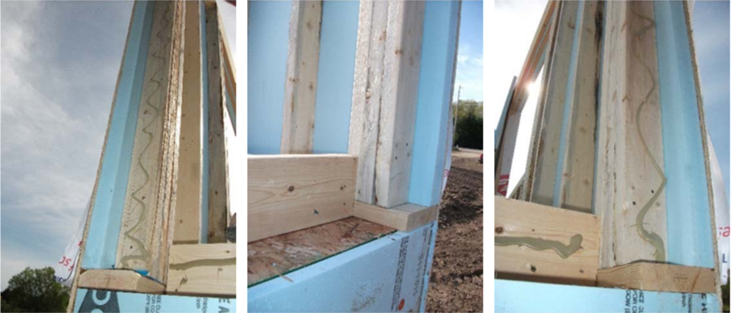
Prepare the ends of the long walls for connection to the short wall. This outside corner configuration places the studs interior to the layer of rigid foam in both directions. Don't forget the continuous bead of caulk for air-sealing.
