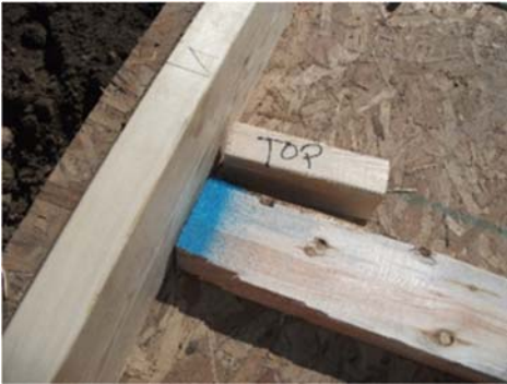
Move the top plate to the center of the floor deck, lay out studs, and cut a spacer from waste 2x4 to measure for 2-in. rigid foam.
