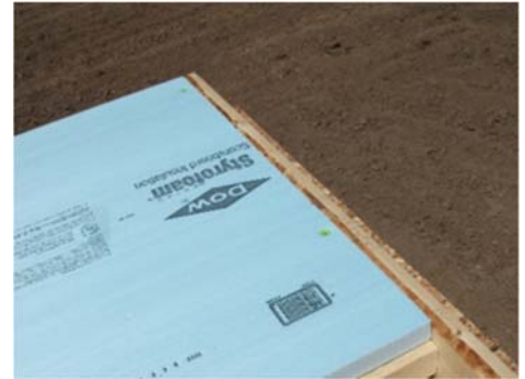
Measure and cut rigid foam for a snug fit between the EP&B wall's top and bottom plates.
