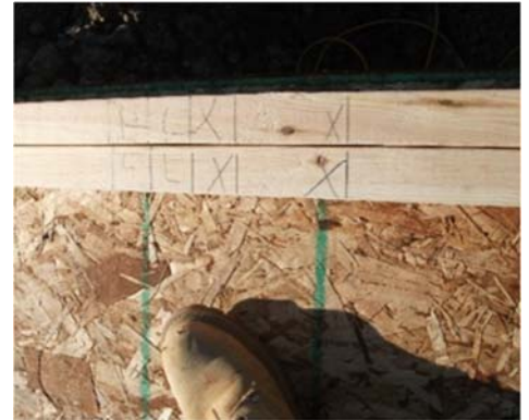
Lay out 2x6 top and bottom plates at deck edge; mark stud locations.
