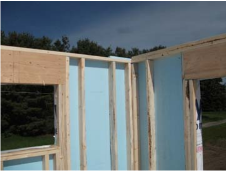
EP&B walls support trusses with WSP nailed to a double top plate.
