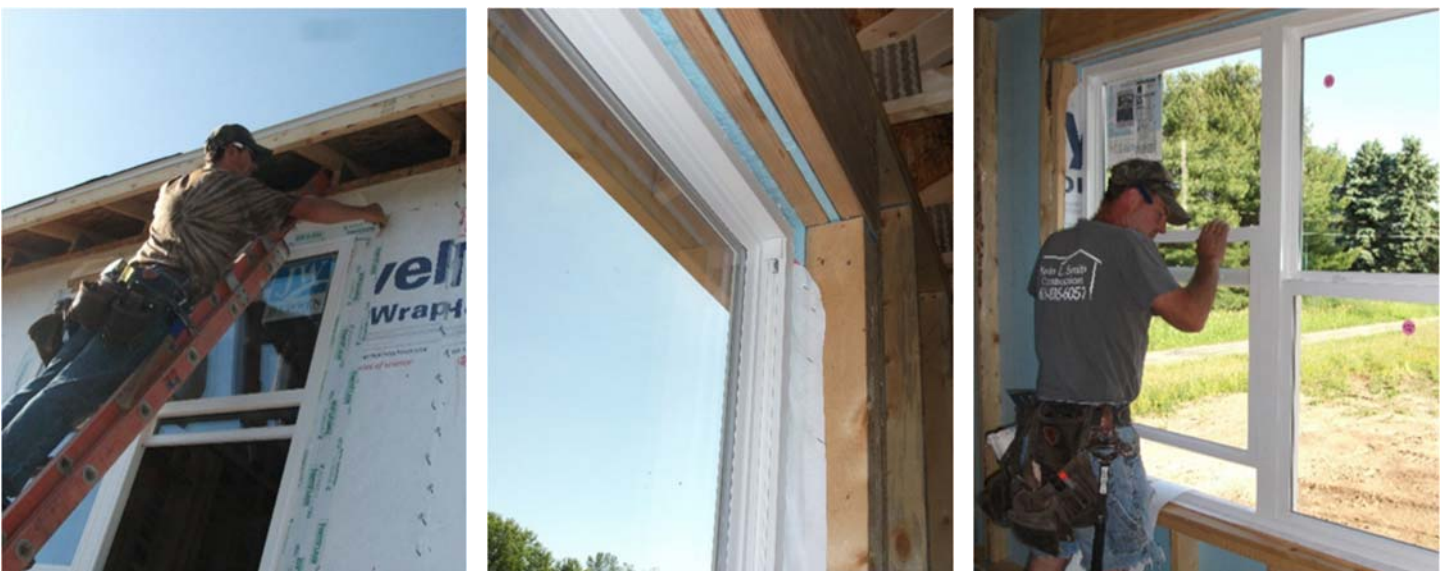
Apply head flashing as the final layer, and then tape the WRB flap over the head flashing.
