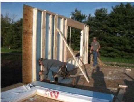
Two adjacent sections of wall must be planned to stagger the vertical joints of the rigid foam and OSB.
