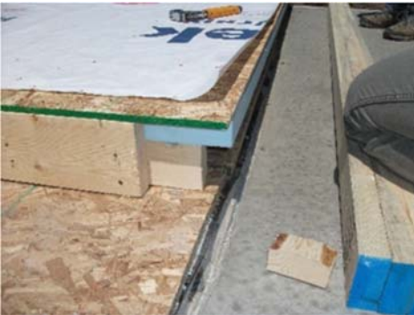
Leave a gap at the top plate for tying adjacent panels together.
