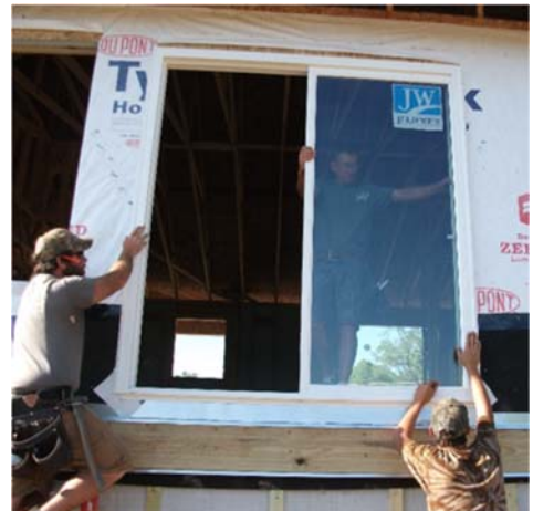
WRB above the door is folded up and away, and is the last waterproofing component to be folded down, as the top "shingle" to prevent bulk water intrusion by shedding water instead of trapping it.
