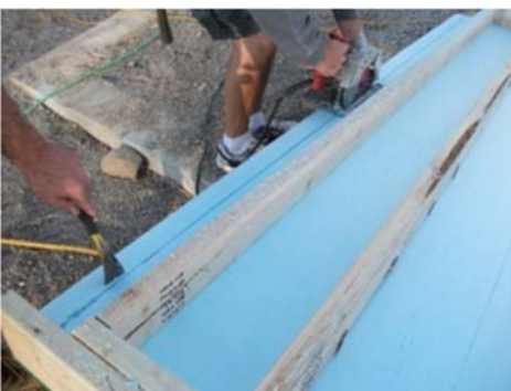
Removing a strip of FPIS to join thermal break at outside corner.
