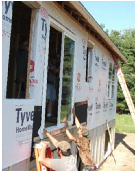
Sills of patio doors require special attention because decks may have standing water.
