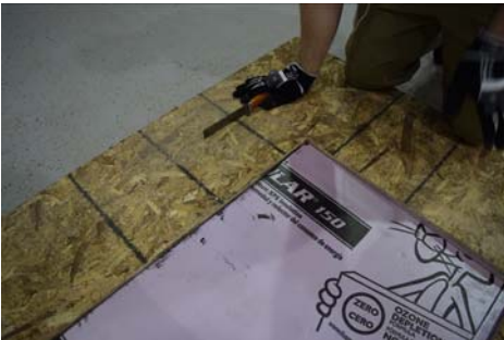
Cut corners of remaining rigid foam with a hand blade or reciprocating saw.
