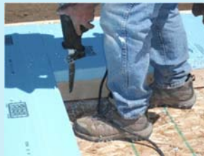
Use the 2x4 framing to guide the reciprocating saw to cut out FPIS.
