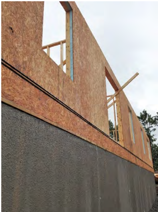
Figure 25. Test Project's Window Openings have 2x4 Framing, Door Openings Have 2x6 Framing
