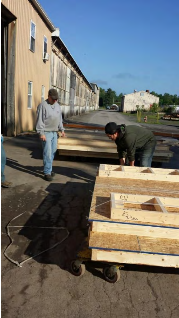
Figure 17. Completed EP&B Wall Panel Bundles at Plant, Ready to be Loaded onto Flatbed Trailer
