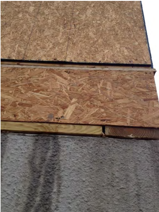
Figure 23. OSB Filler over Rim (gap was considered too small for FPIS filler)
