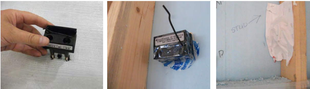
Figure 72. Sensor cabinets are protected from intrusion of moisture and debris with WRB tape
