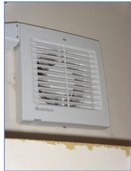
Figure 45. Interior Exhaust Fan Grill
