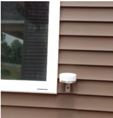
Figure 7. Exterior sensor attached to the cladding
