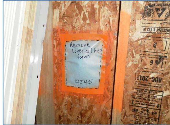
Figure 4. Sensor Installed in OSB Sheathing That Will Not be Foamed Over in This Cavity
