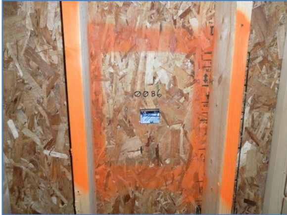
Figure 3. Sensor Installed in OSB Sheathing That Will be Foamed Over in This Test House
