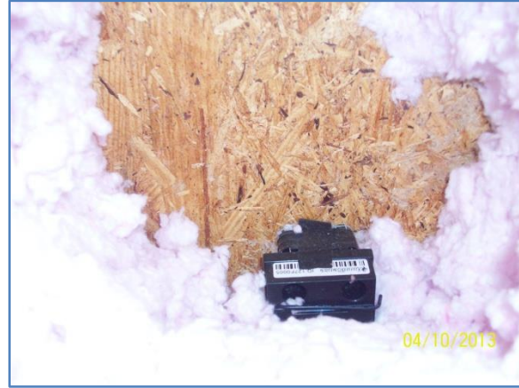
Figure 54. Moisture Sensor Located
