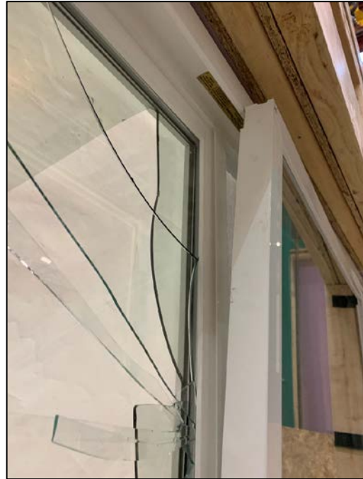
Figure 39. Window Sash Popping Out of Frame
