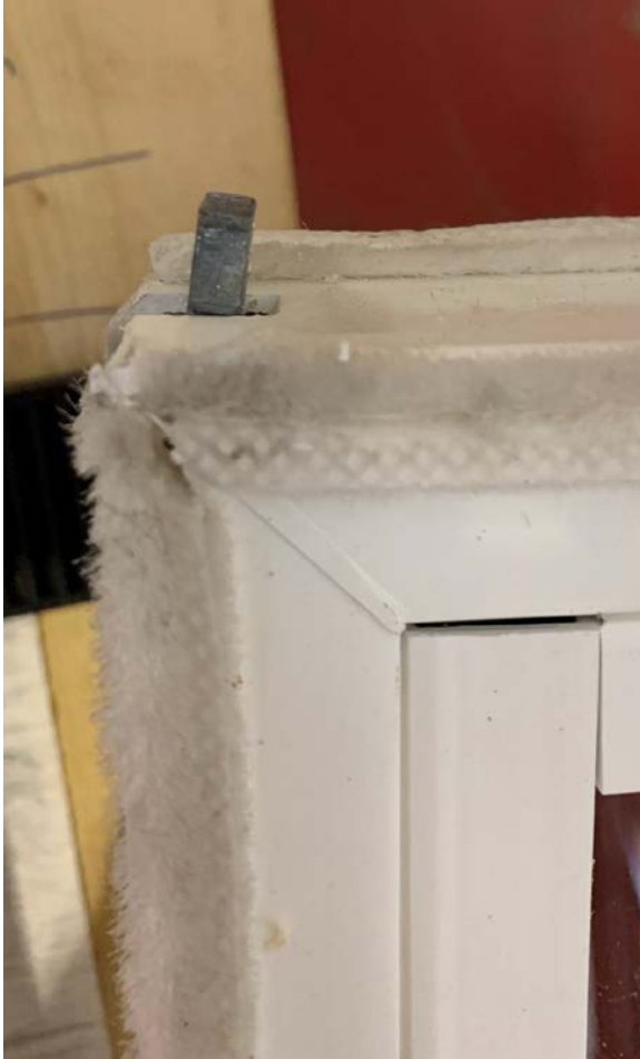
Figure 18. Sash Hook Slightly Bent
