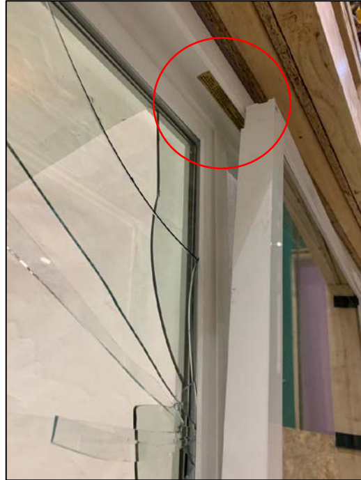
Figure 20. Window Sash Popping Out of Frame
