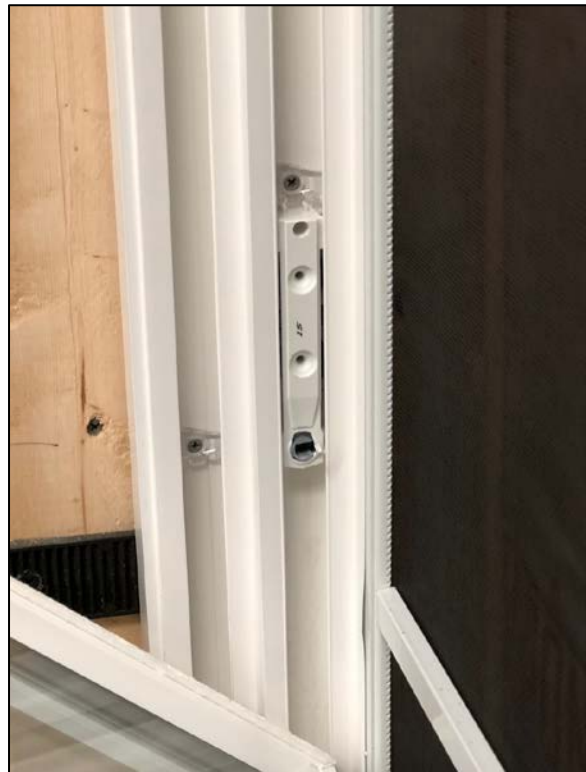
Figure 17. Window Sash Popped Out from Counterbalance Mechanism
