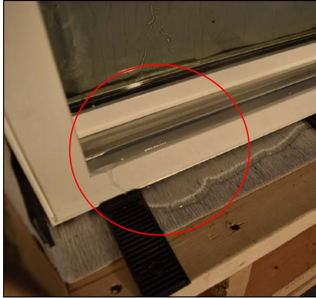
Figure 14. Water Pooling and Overflowing During the Water Test
