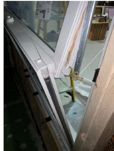
Figure 32. Window Sash Damage
