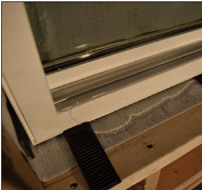
Figure 40. Water Pooling and Overflowing During the Water Test
