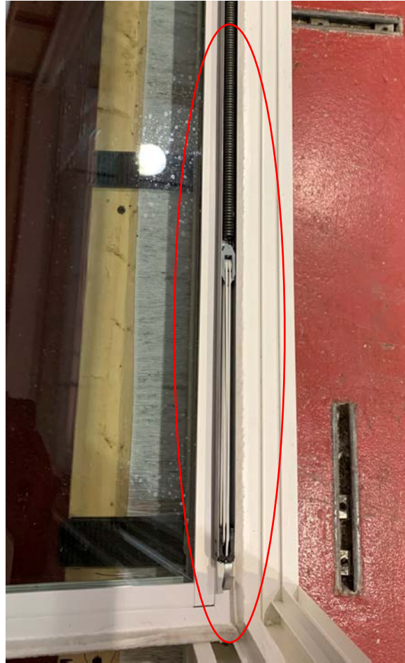
Figure 19. The Counterbalance Mechanism Fell When the Window Was Inspected.
