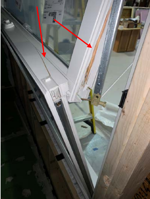
Figure 15. Window Sash Damage
