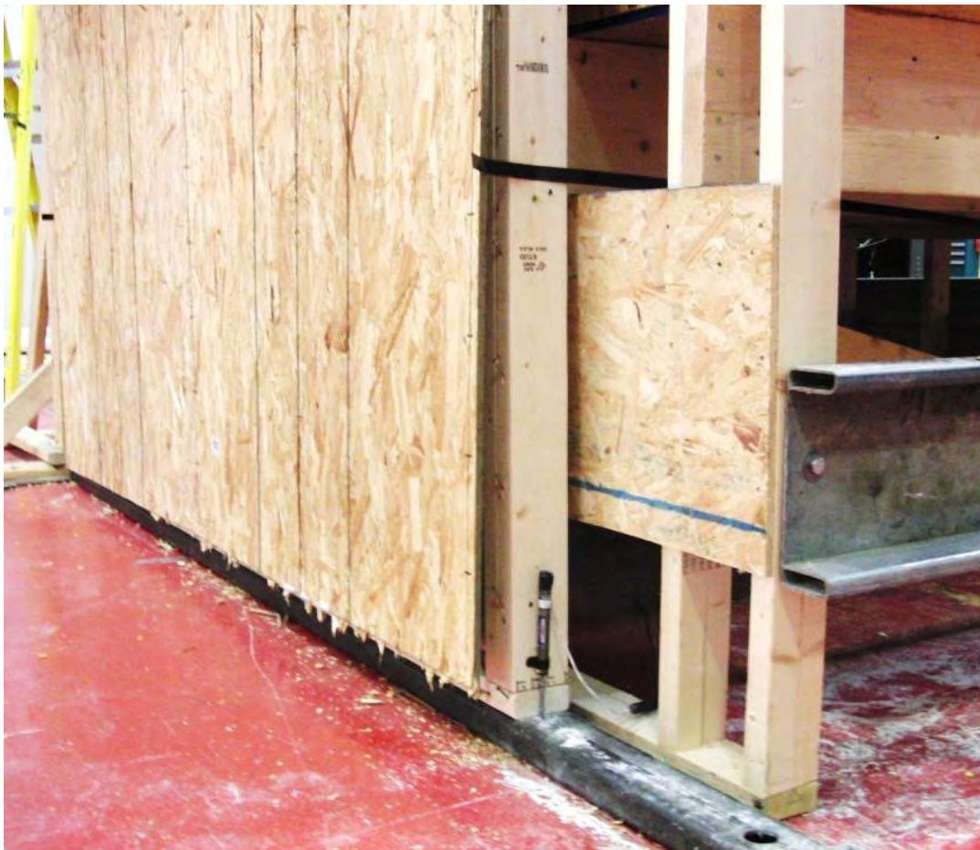
Figure 13 – Fastener pull-through failure mode of Test C and Test D
