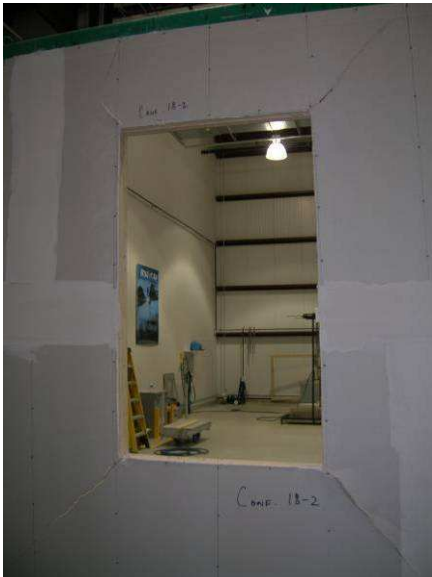
Figure 19 – Configuration 13 (Cracks at window)
