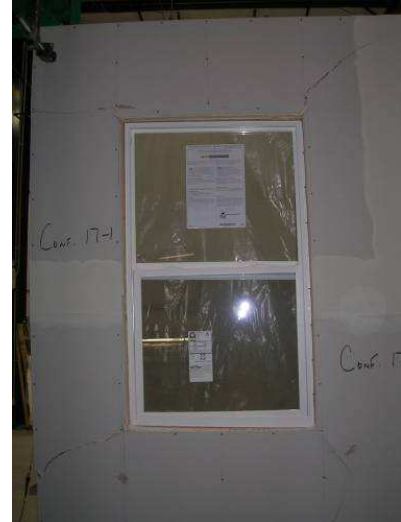
Figure 28 – Configuration 18 (Gypsum cracking)
