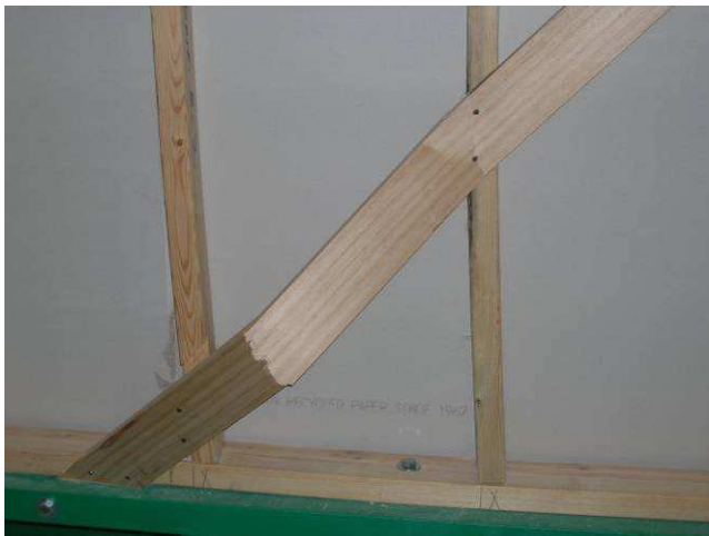
Figure 13 – Configuration 6 (Let-in brace buckling)
