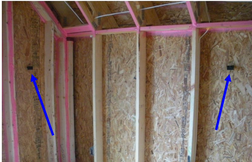
Figure 6. OmniSensors Installed in Wall Cavities
