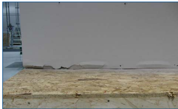
Figure 11. Example gypsum board damage
