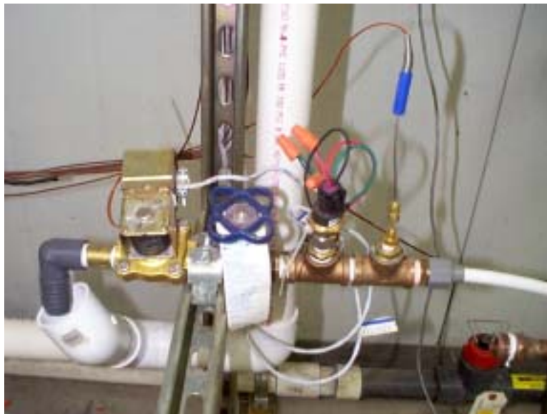
Figure 6. Outlet measurement system
