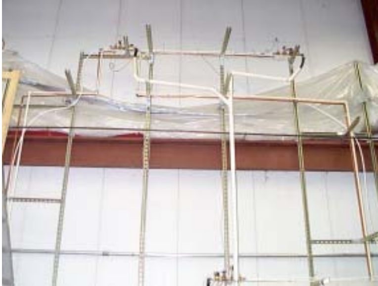
Figure 3. Partial piping system showing PEX and copper distribution systems, drains, and outlet measurement systems
