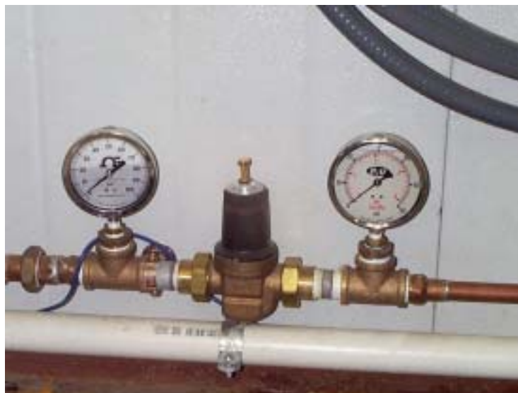
Figure 5. Inlet pressure monitoring and regulation system
