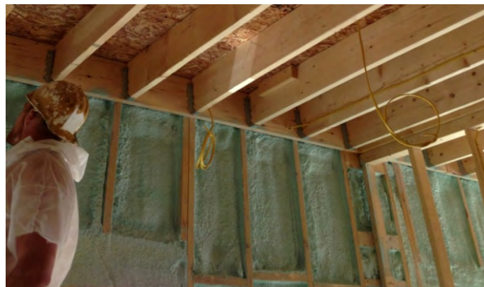
Figure 7. Exterior wall air sealing used at HV
