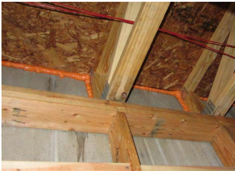
Figure 9. Air sealed sheetrock smoke curtain used at demising wall of SH
