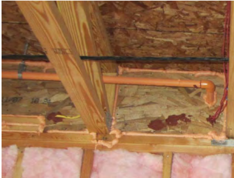
Figure 8. Air sealed plywood smoke curtain used at demising wall of CV
