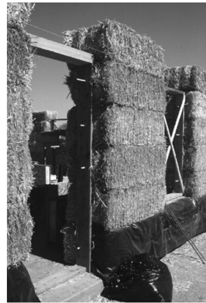
Straw-bale wall construction achieves significant insulation levels through density of organic material. Bales are easily assembled on site and require minimal building skills.
