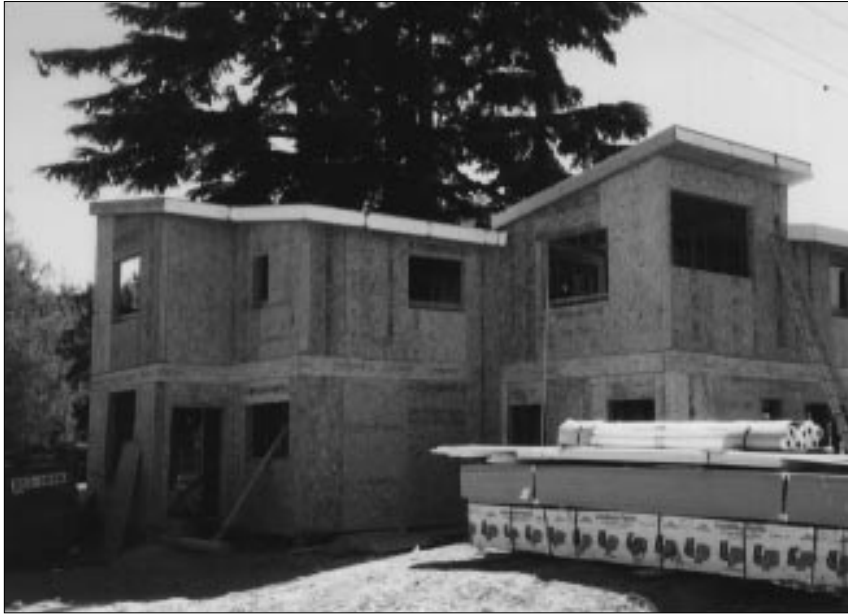
The City Life project displays different construction techniques. Duplex unit is of SIP technology, with townhouse and courtyard units are of conventional site-built construction. All are energy efficient.
