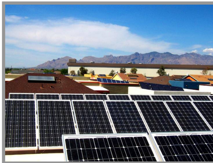
Figure 7 - ZEH2 PV System
