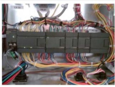
Figure 7 Original PLC used as the control module of the heat pump.
