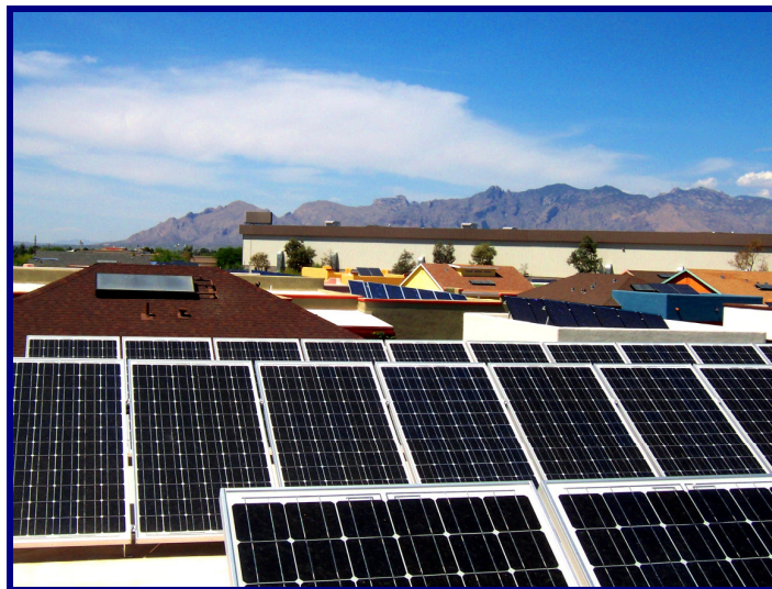
Figure 2. APdS PV Systems
