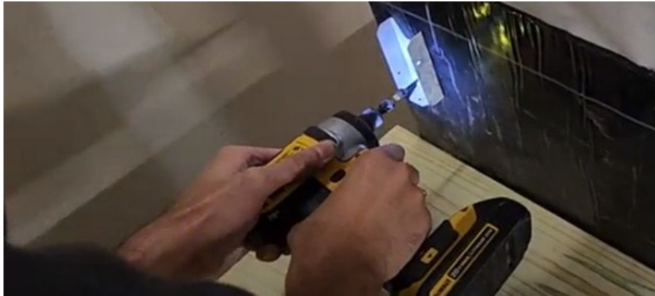
Figure 70. Mount Rail Bracket on Exterior Wall
