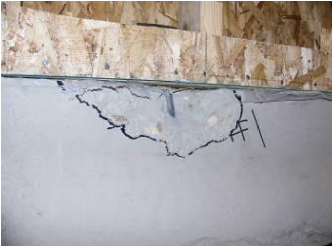
Figure 27 – Large spall in full-scale shear wall specimen during cyclic testing (sheathing removed post-test to allow for inspection)
