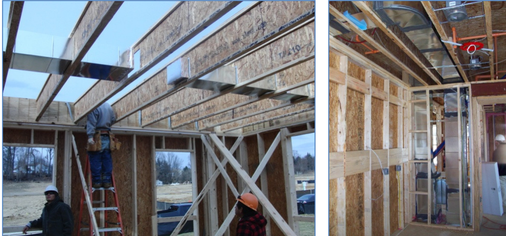
Figure 3. Supply Trunk through Floor Joists & Central Duct Chase
