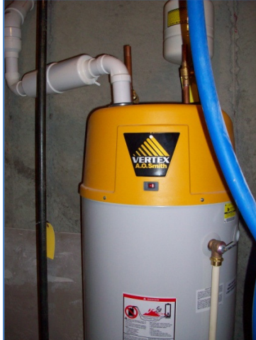
Figure 16. High Efficiency Water Heater
