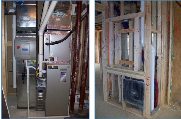
Figure 14. Furnace and First Floor Return Grille at Central Chase
