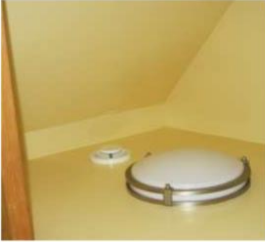
Figure 12: None of the flow hoods would fit into the space adjacent to this bathroom ERV inlet, it went unmeasured
