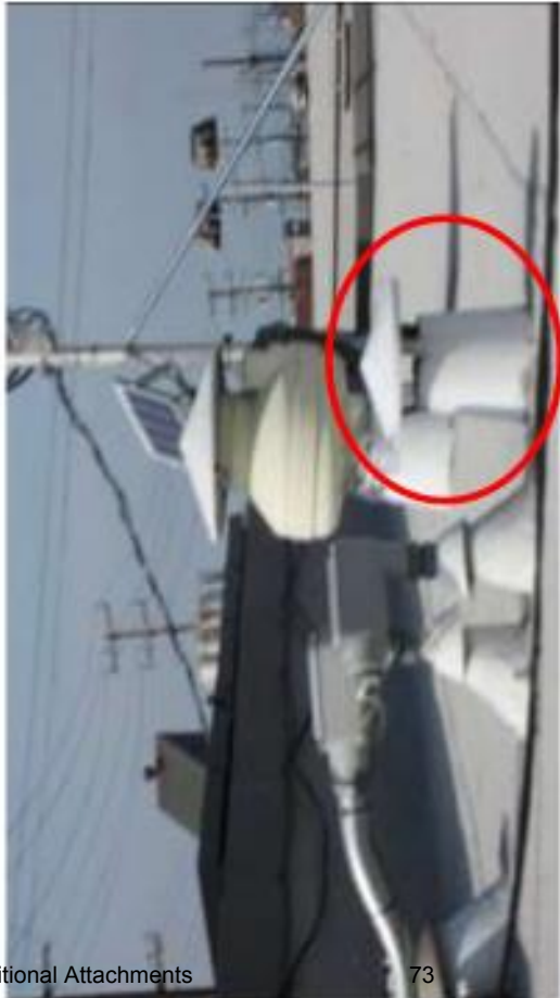
Figure 16: We located FH6's range hood outlet (circled) on its roof, but for safety reasons did not try to measure its flow
