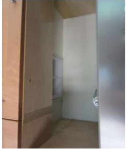
Figure 14: The refrigerator has to be pulled out to measure this kitchen ERV inlet, and even then, the uneven surface prevented measurement with most of the flow hoods
