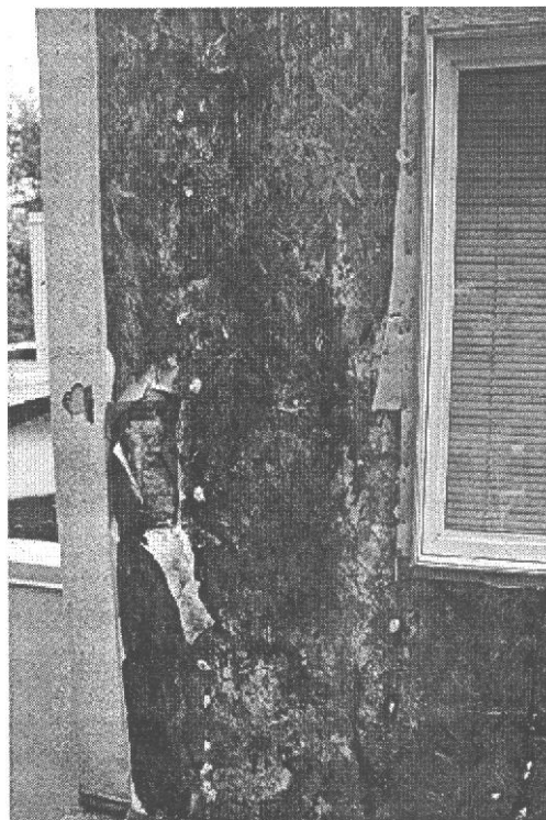
Figure 1. —Extensively decayed OSB wall sheathing on a single-family residence in Middleton, Wisconsin, less than a decade old. Sheathing deterioration was associated with water intrusion around cladding details.
