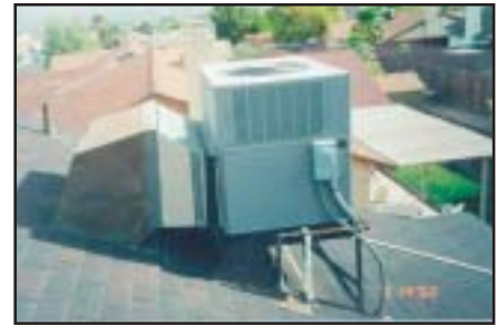
Figure 16 New 12 SEER Puron HVAC System
