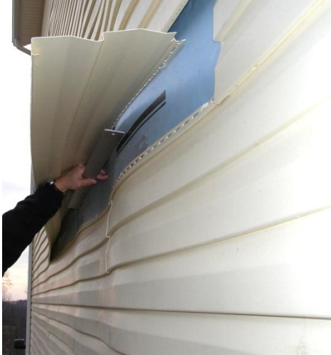
Figure 3 – Wall with buckled OSB panels (siding removed exposing water resistive barrier)
