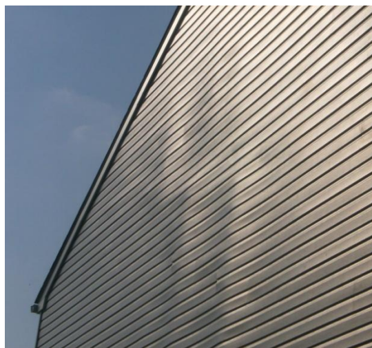
Figure 2 – Wavy siding due to buckled OSB panels on a side wall of a house
