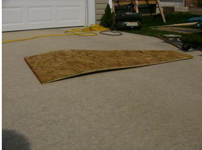
Figure 4 – Removed buckled OSB panel
