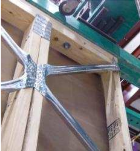
Figure 18 – Combined buckling and withdraw failure at leading edge of wall (Specimen K)
