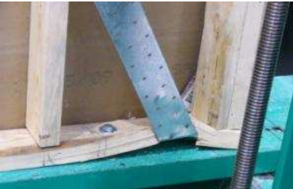
Figure 24 – Flexural and cross grain failure of bottom plate (Specimen N)
