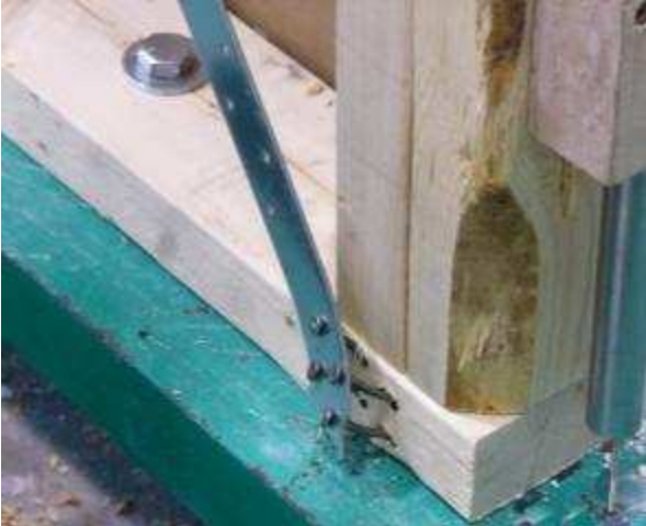
Figure 22 – Withdrawal failure of metal brace (Specimen M)
