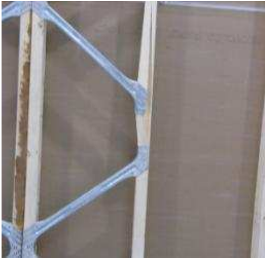
Figure 20– Splitting failure of stud (Specimen K)
