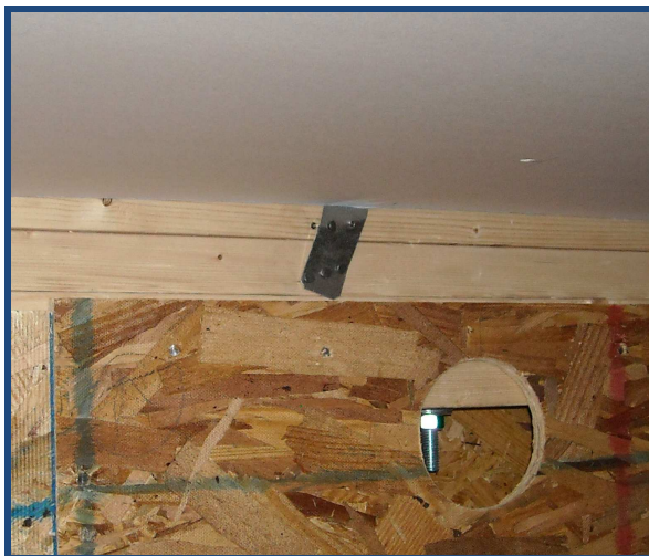
Figure 13 – Rotation of hurricane clip at failure (Specimen A)
