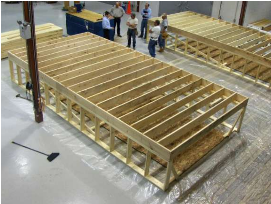
Figure 1: View of the floors from the observation deck level prior to the subflooring installation trials
