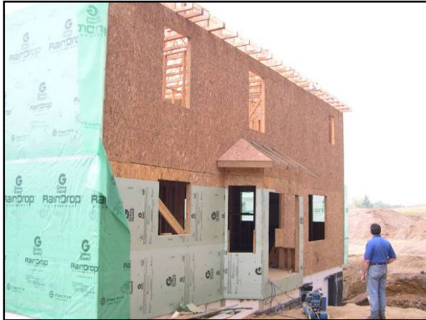
Figure 14. All Exterior walls are fully sheathed With 7/16” OSB and over-sheathed with 1”XPS foam sheathing.
